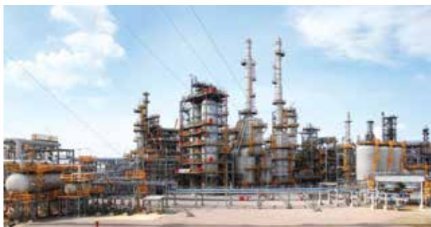
ExxonMobil's Singapore hydrotreater helps produce ultra-low sulphur diesel and contributes to lower vehicle emissions
